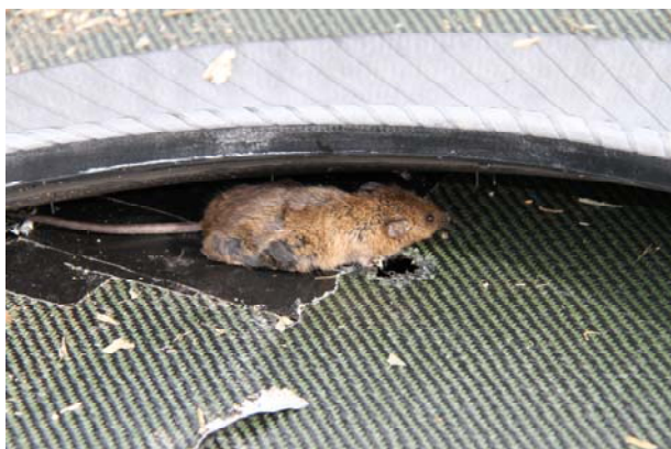
Mice damage to silage pit cover
