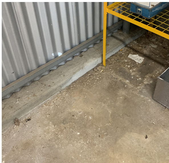
Figure 8. Bunding around a chemical storage shed.
